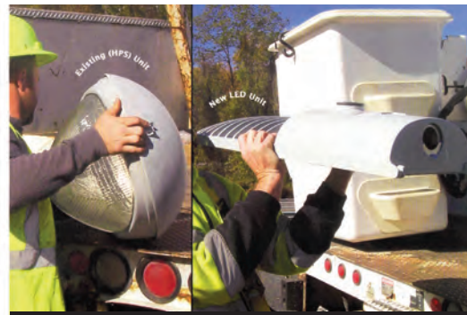
I-83 Warren Road LED Roadway Lighting Pilot Century Engineering Inc.
