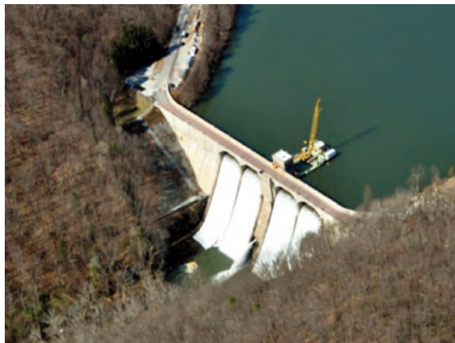
Alvi Associates Gatehouse Anchorage System for Prettyboy Dam (Baltimore, MD)
