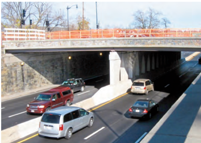
Greenhorne & O'Mara Reconstruction of Eastern Avenue Bridge over Kenilworth Avenue, N.E. (Washington, DC)
