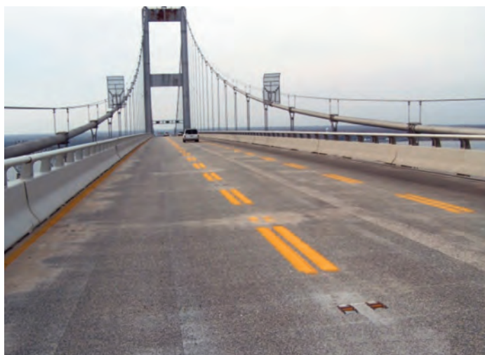
URS Corporation Deck Replacement of Westbound Suspension & Through Truss Spans & Miscellaneous Repairs (Annapolis, MD)
