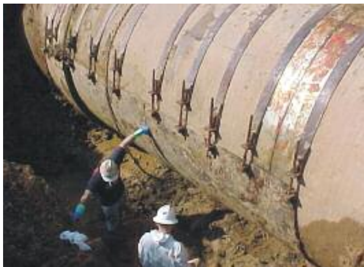
Honor Award - Gannett Fleming, Inc. - Emergency and Long-Term Repair of the Southwest Diversion Pressure Sewer
