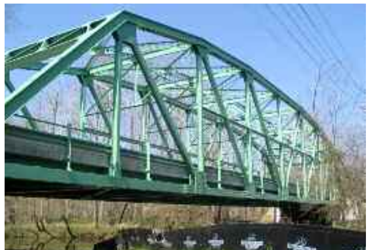
HONOR AWARD IN STRUCTURAL SYSTEMS - MD 214 over Patuxent River (Davidsonville, MD) - Alvi Associates
