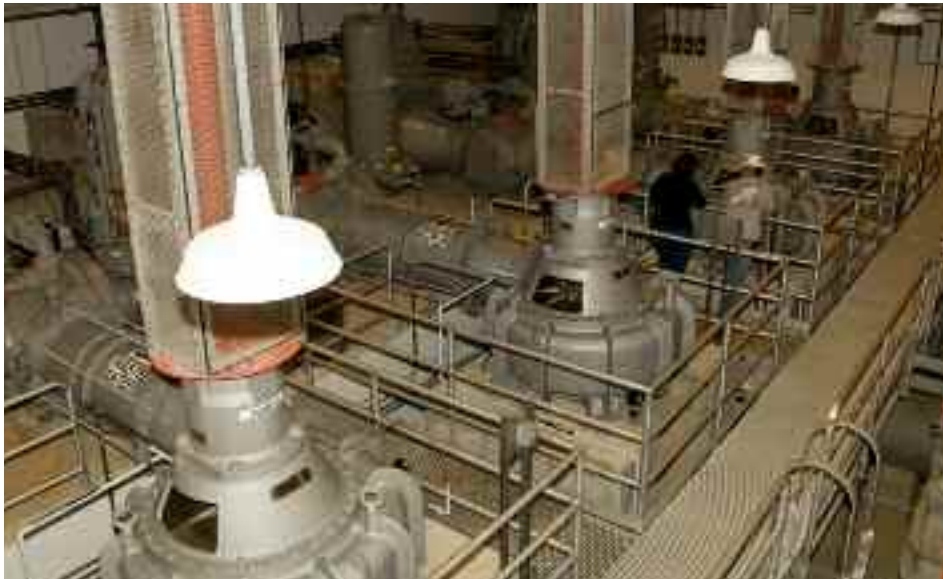
HONOR AWARD IN ENVIRONMENTAL, WATER AND WASTEWATER, AND WATER RESOURCES - Stemmers Run Relief Wastewater Pumping Station, Force Main, and Relief Sewer (Baltimore Co., MD) – Rummel, Klepper & Kahl (RKK)
